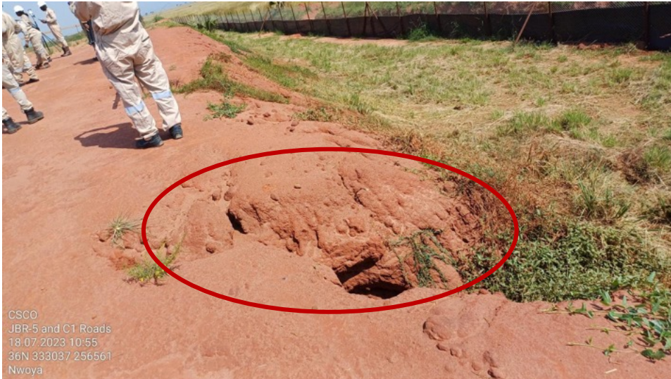
Figure 16: Marks of erosion (Gullies) exhibiting signs of loss of aesthetics at the JBRI-5 well pad site.
