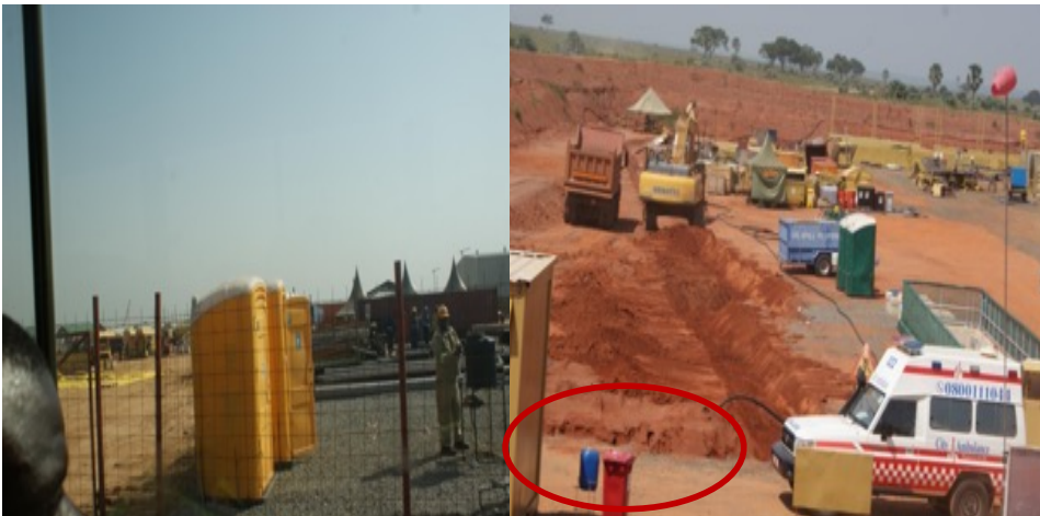
Figure 4: Pictures showing sanitary facilities such as water points for hand washing and movable toilets on sites.
