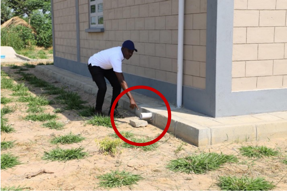
Figure 12: Gutters from the roof at one of the newly constructed Tilenga RAP2-5 Resettlement houses (in the encirclement) not connected to any outfall drainage system for safe disposal of storm water.
