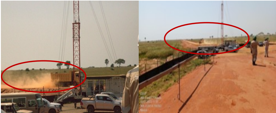
Figure 11: Dust emission and uncovered contractor's truck along C1 road near JBRI-5 well-pad construction area.
